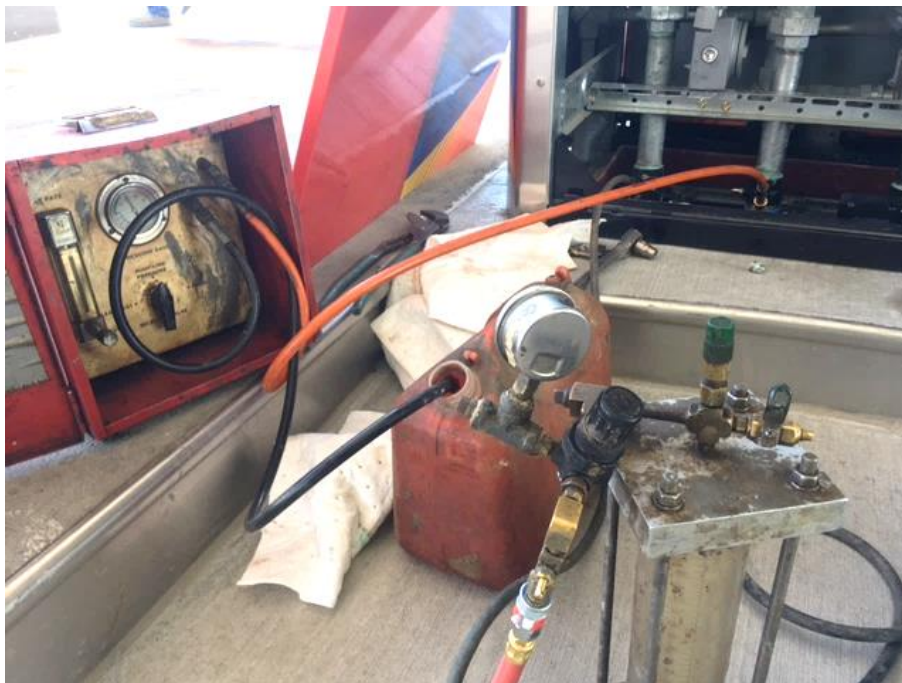
Fig. 6 - line & automatic line leak detector (ALLD) testing
